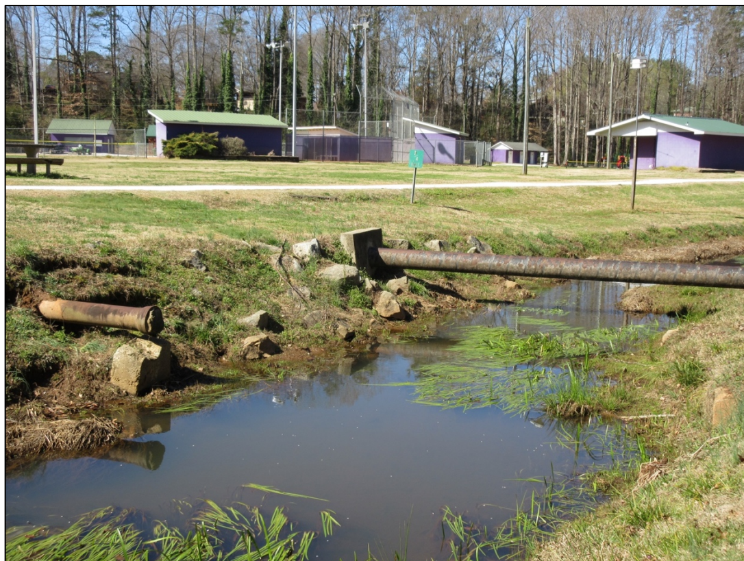
Fig.18. Previously sealed and replacement sewer lines hover just a few feet over unnamed tributary leading to Cane Creek, which runs through Sertoma Field, Walhalla, SC.
