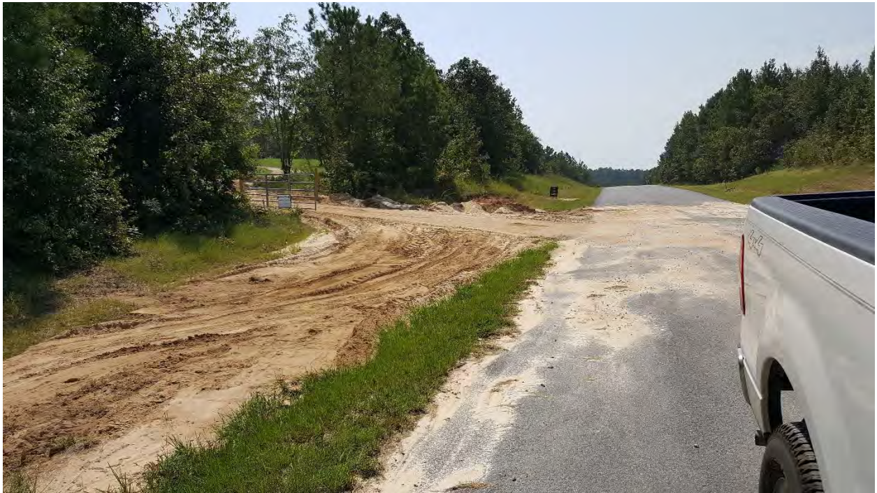
Figure 17. Tod's Hill subdivision in need of stabilized construction entrance.
