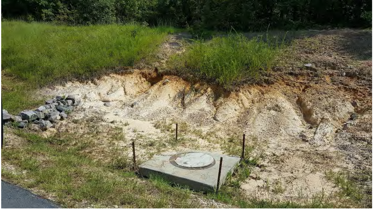
Figure 16. Tod's Hill subdivision in need of sediment and erosion control measures.
