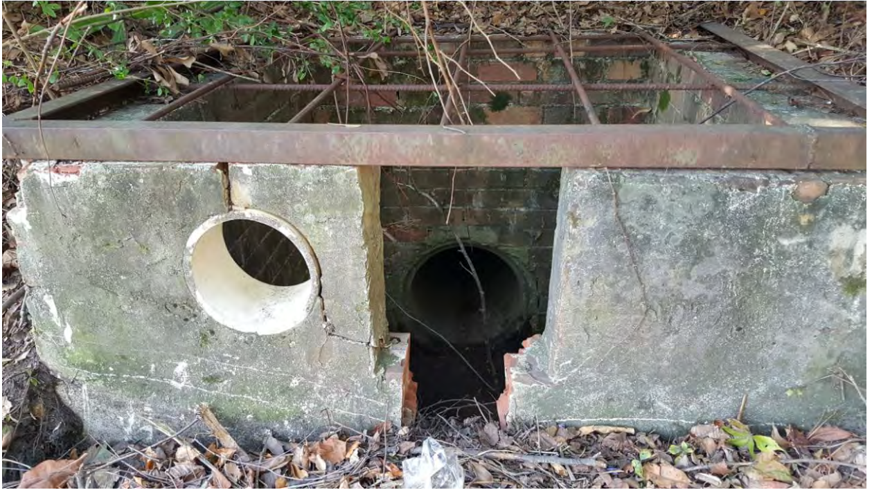
Figure 23. Gas station's stormwater infrastructure
