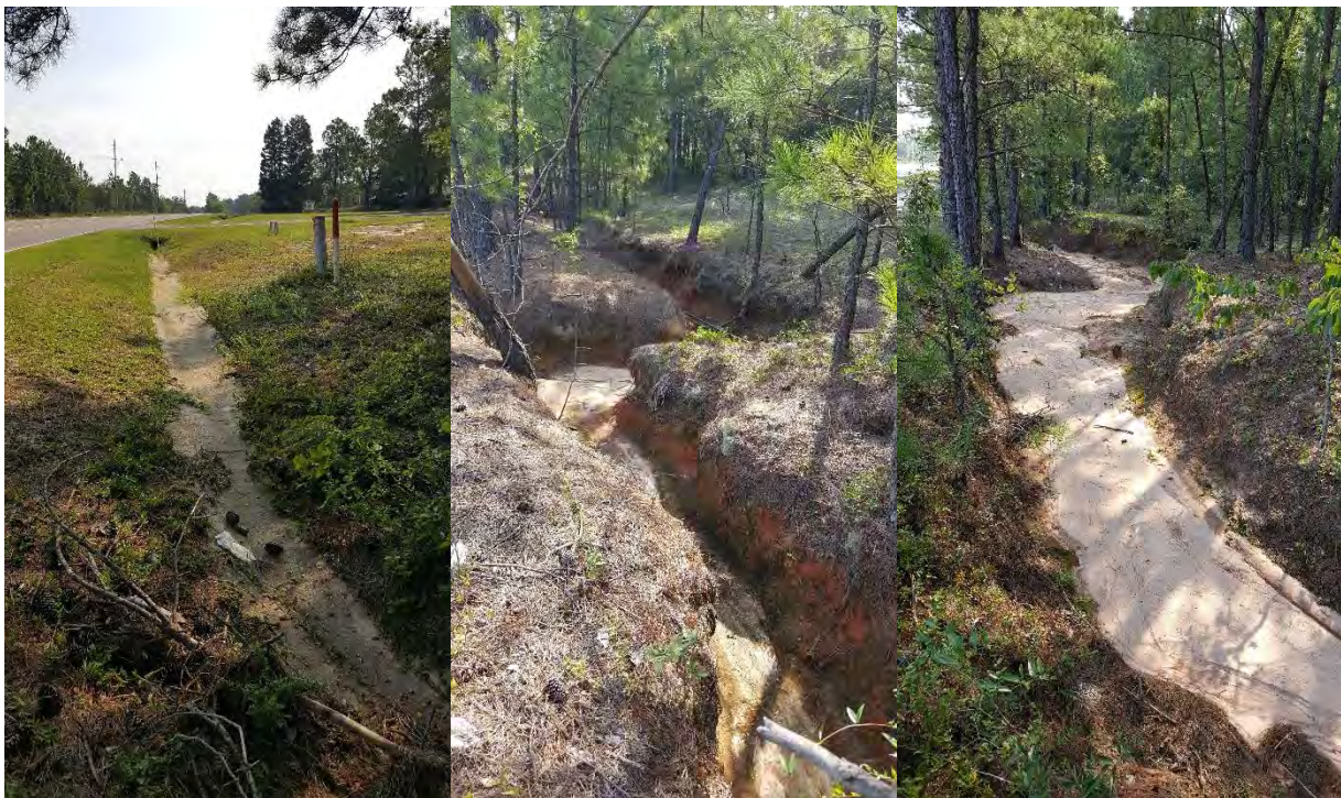
Figure 11. Eroded SCDOT Ditch down gradient from Industrial Service Corp. along Windham Blvd.
