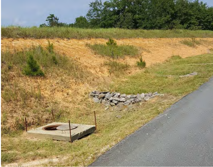
Figure 18. Tod's Hill subdivision in need of sediment and erosion control measures.
