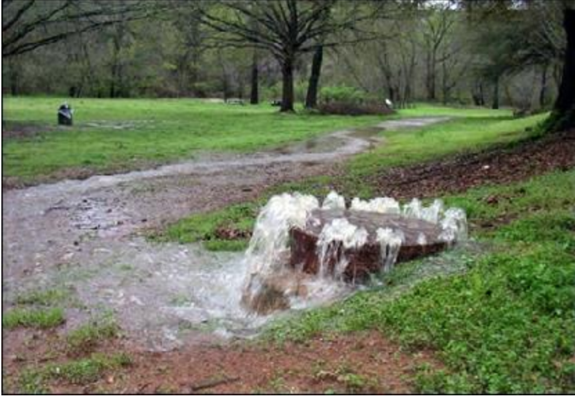
FIGURE 31. SANITARY SEWER OVERFLOW
