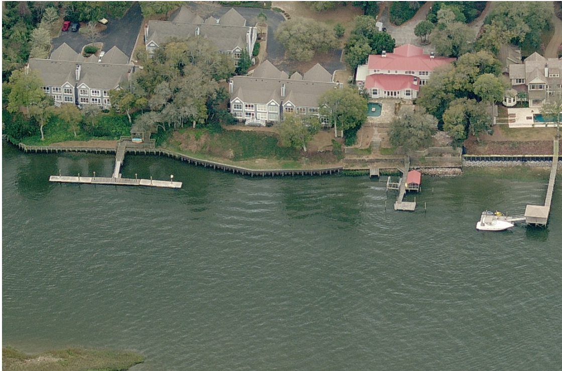
Figure 9: Estuarine shoreline erosion control structures near Charleston, SC. Many stretches of tidal creek shorelines in South Carolina have been armored with a variety of structures including wooden bulkheads and rock revetments.
