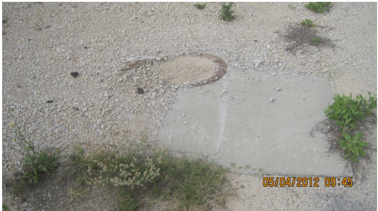
Photo 4: Partial view of fill port for closed-in-place diesel underground storage tank (UST).
