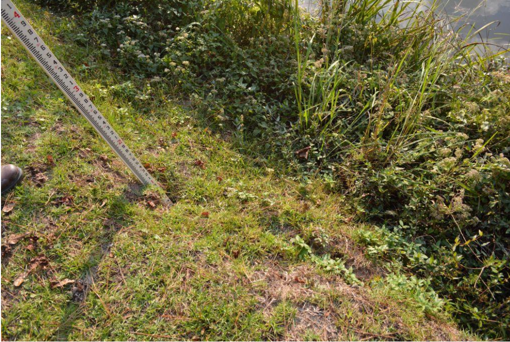
Photo 3: Slough on upstream face
