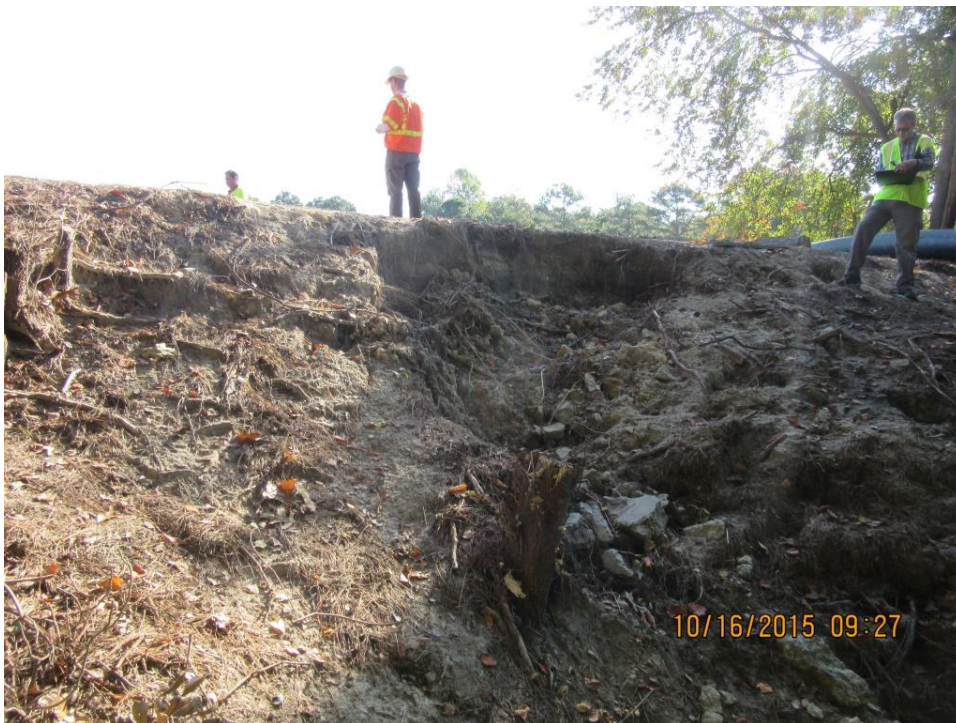
Photo 6: View of slough of embankment from downstream
