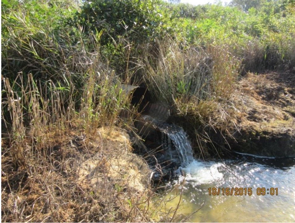
Photo 5: Service spillway outlet pipe. Note minor erosion around the pipe.
