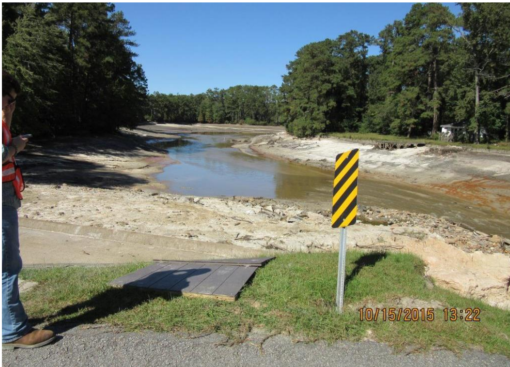
Photo 4: Upstream view; concrete approach slab of right auxiliary spillway is in the foreground
