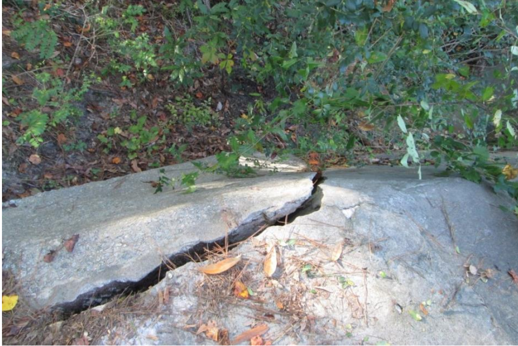
Photo 9: Vertical crack/slabbing in left abutment of lower stone dam
