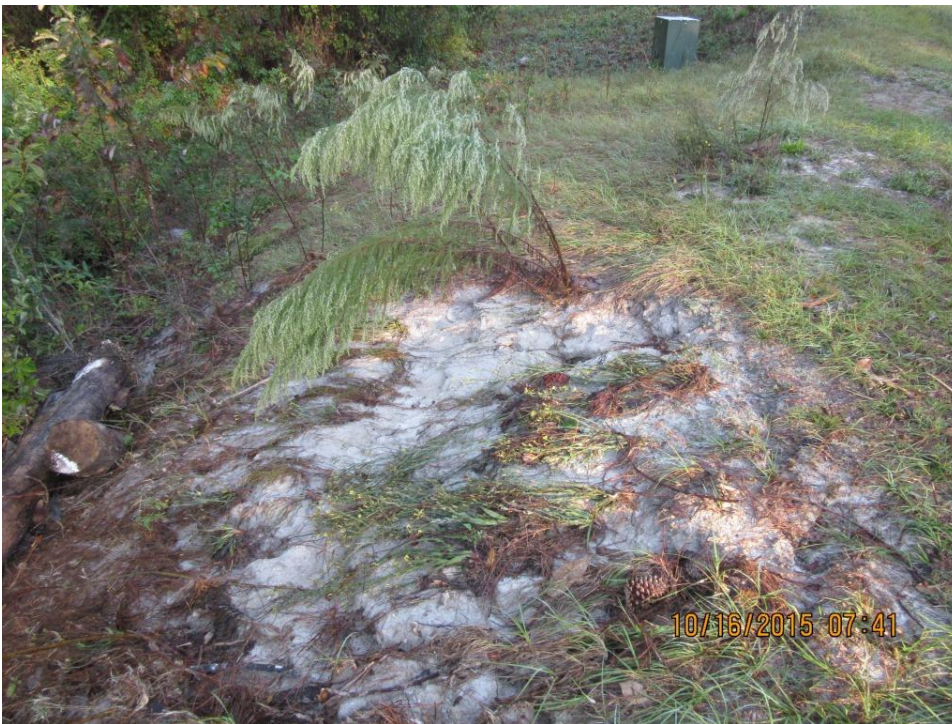
Photo 2: Minor erosion of the left downstream embankment.
