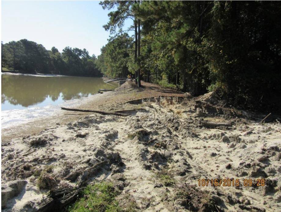
Photo 3: View of approach to the emergency channel that was excavated at the right abutment during the flood to convey water downstream
