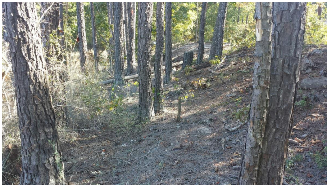
Photo 2: Tree growth on upstream embankment slope
