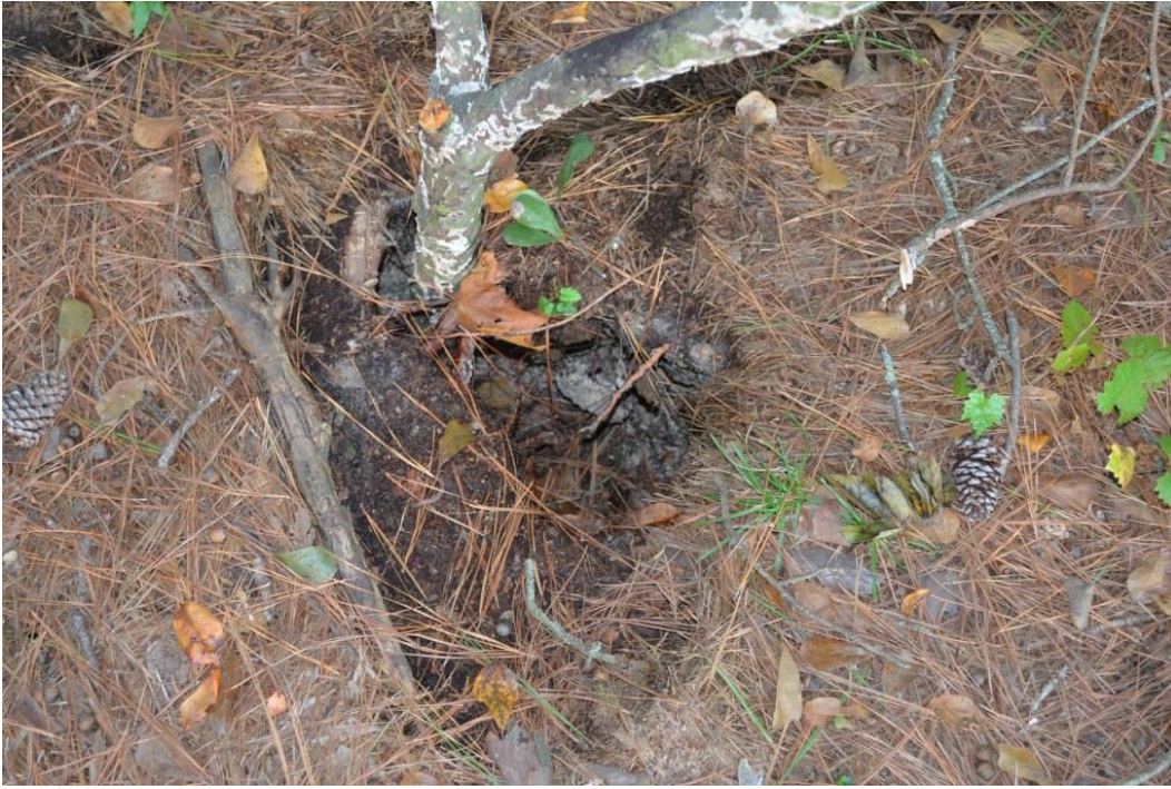
Photo 4: Depression on embankment crest
