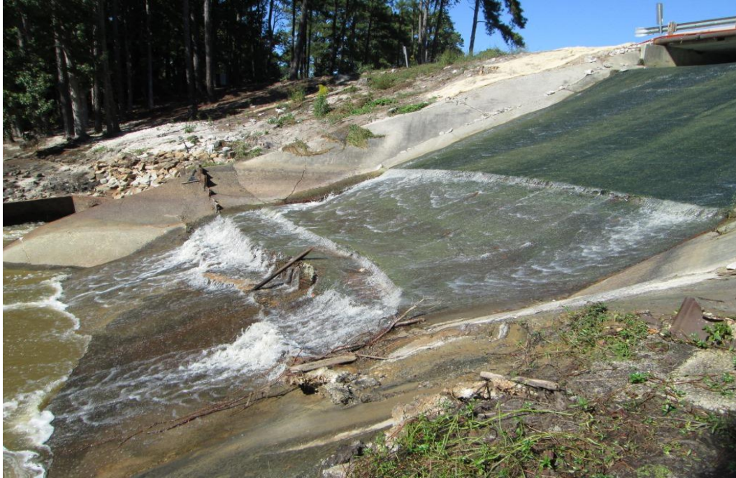
Photo 7: View of sheetpile at toe of auxiliary spillway; note cracks in concrete surface adjacent to sheetpiles
