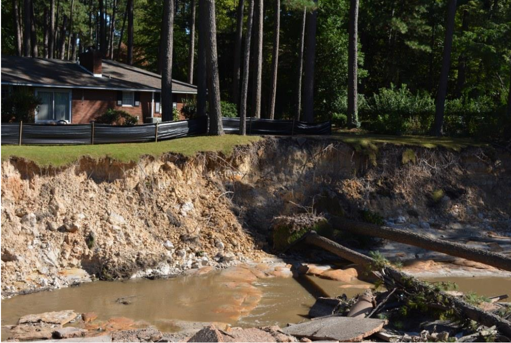
Photo 5: Erosion along the left side of the auxiliary spillway, looking downstream from the bridge
