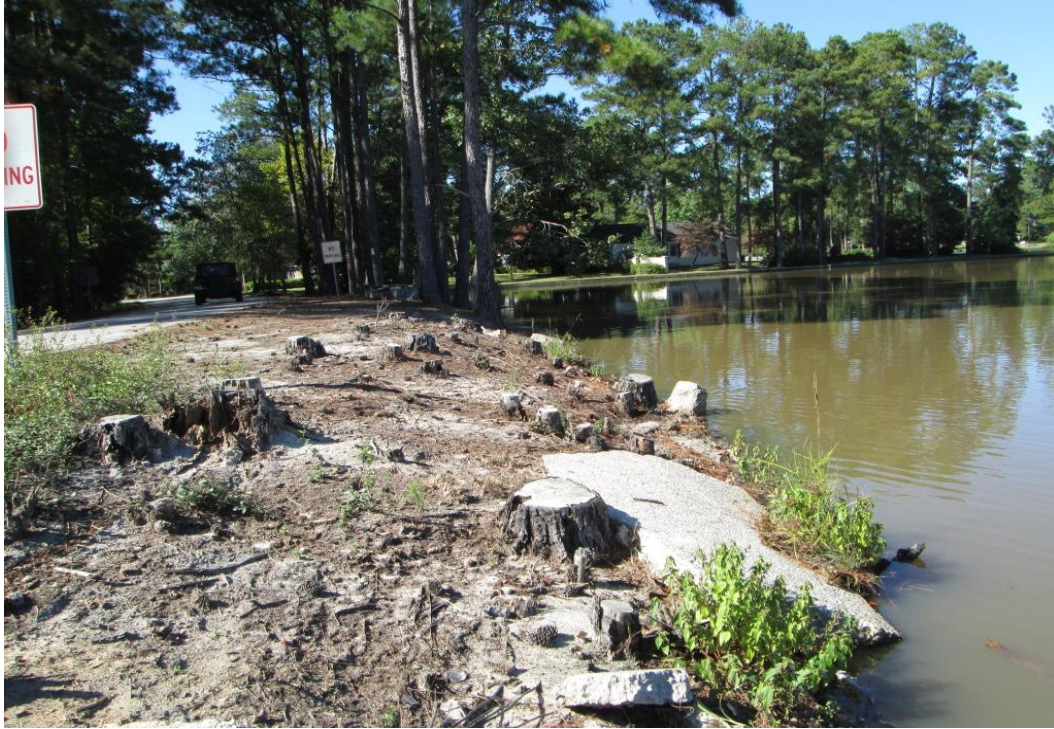
Photo 3: Upstream slope of right embankment with tree stumps and mature trees
