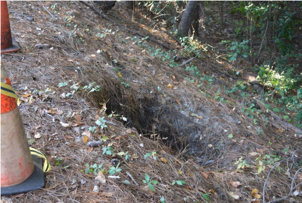
Photo 8: Depression on downstream slope above spillway alignment
