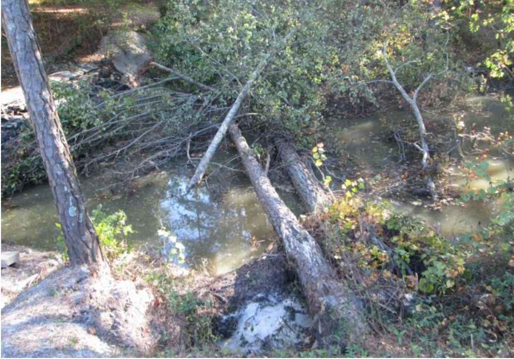
Photo 11: Felled trees in auxiliary spillway between upper and lower masonry stone dams
