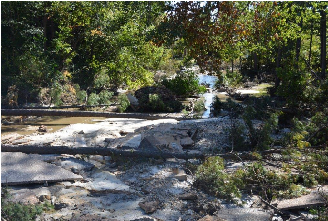
Photo 6: View of the auxiliary spillway looking downstream of bridge; concrete debris is seen in the foreground
