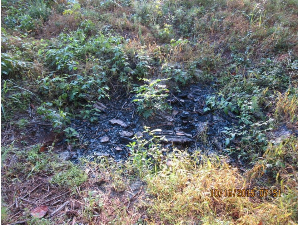
Photo 3: Depression at toe of embankment
