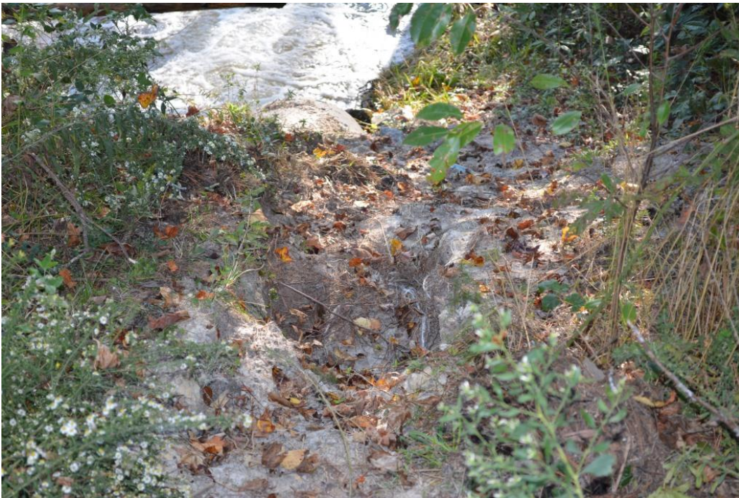
Photo 4: Scour on downstream embankment slope
