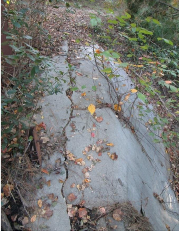
Photo 7: Crack in left abutment of the upper masonry stone dam
