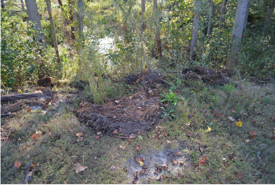
Photo 3: Debris accumulation on downstream embankment slope due to overtopping
