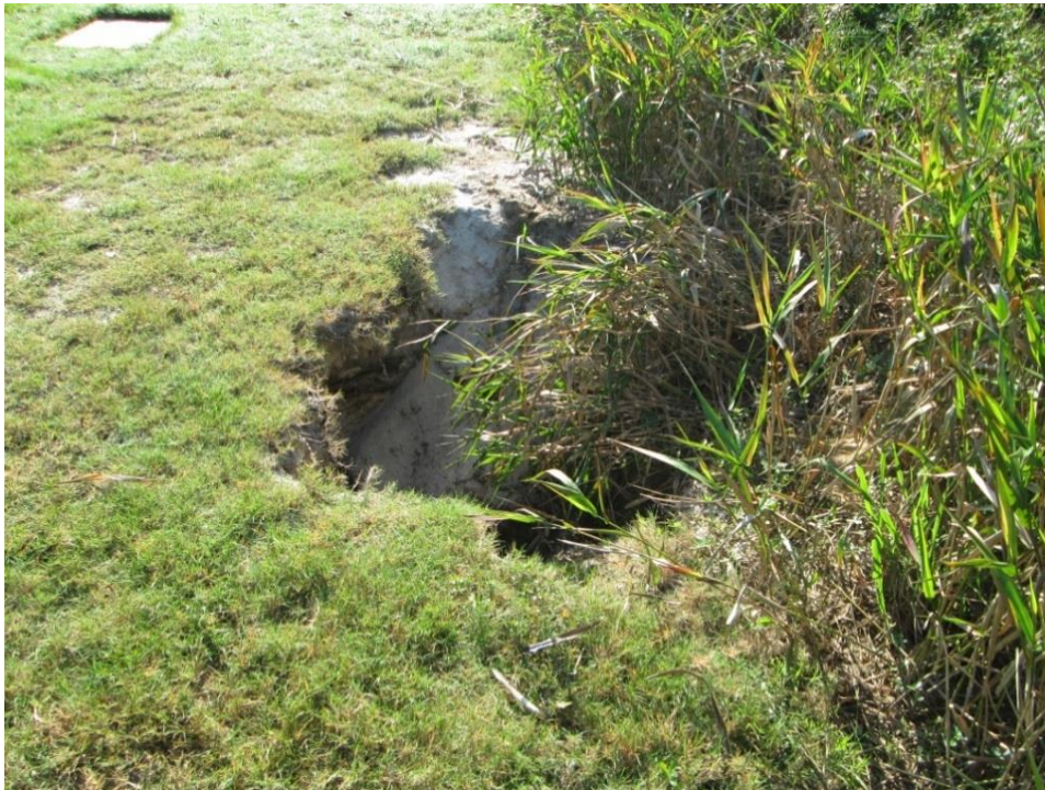
Photo 6: Erosion on downstream slope of embankment, approximately 30 feet upstream of the service spillway outlet
