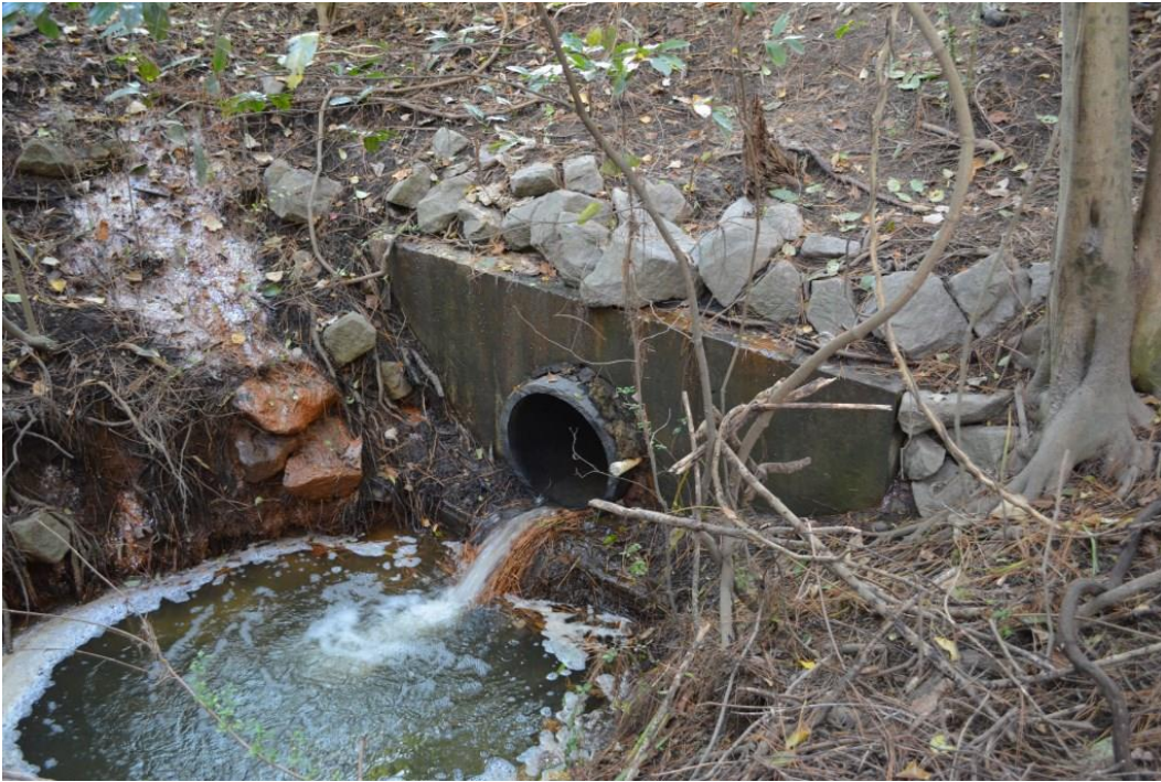
Photo 6: Service spillway outlet pipe and seepage
