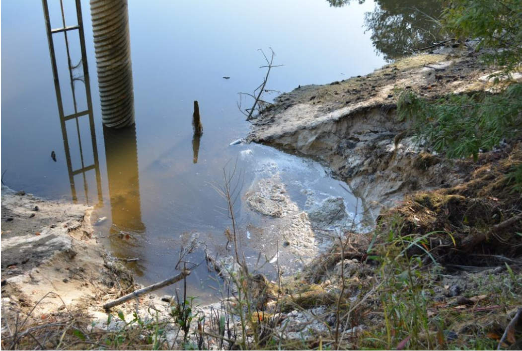
Photo 7: Upstream slope failure along service spillway alignment
