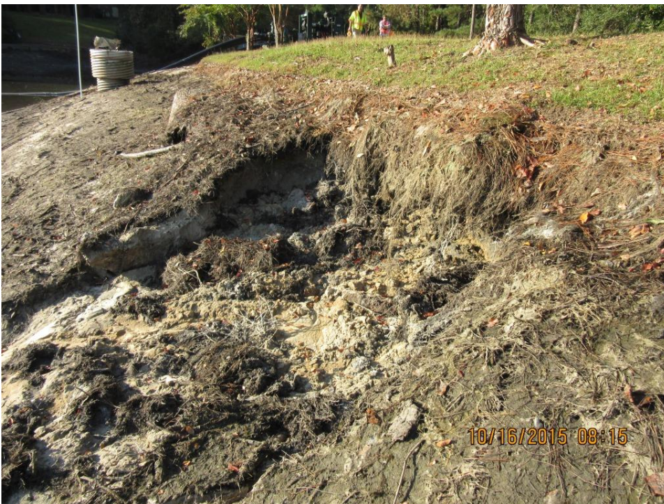
Photo 2: Upstream embankment slope slough
