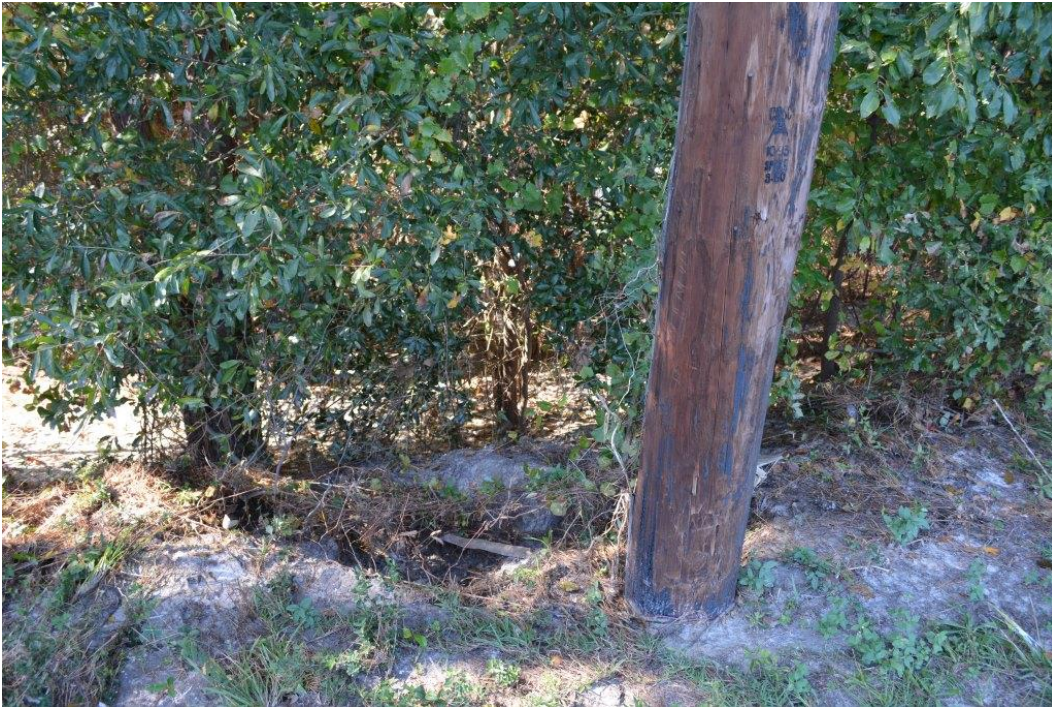
Photo 4: Slough and debris on downstream slope
