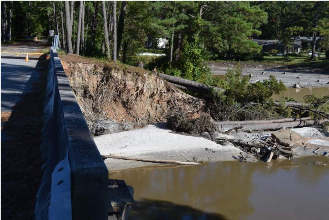
Photo 2: View of eroded embankment at left abutment of the auxiliary spillway looking downstream
