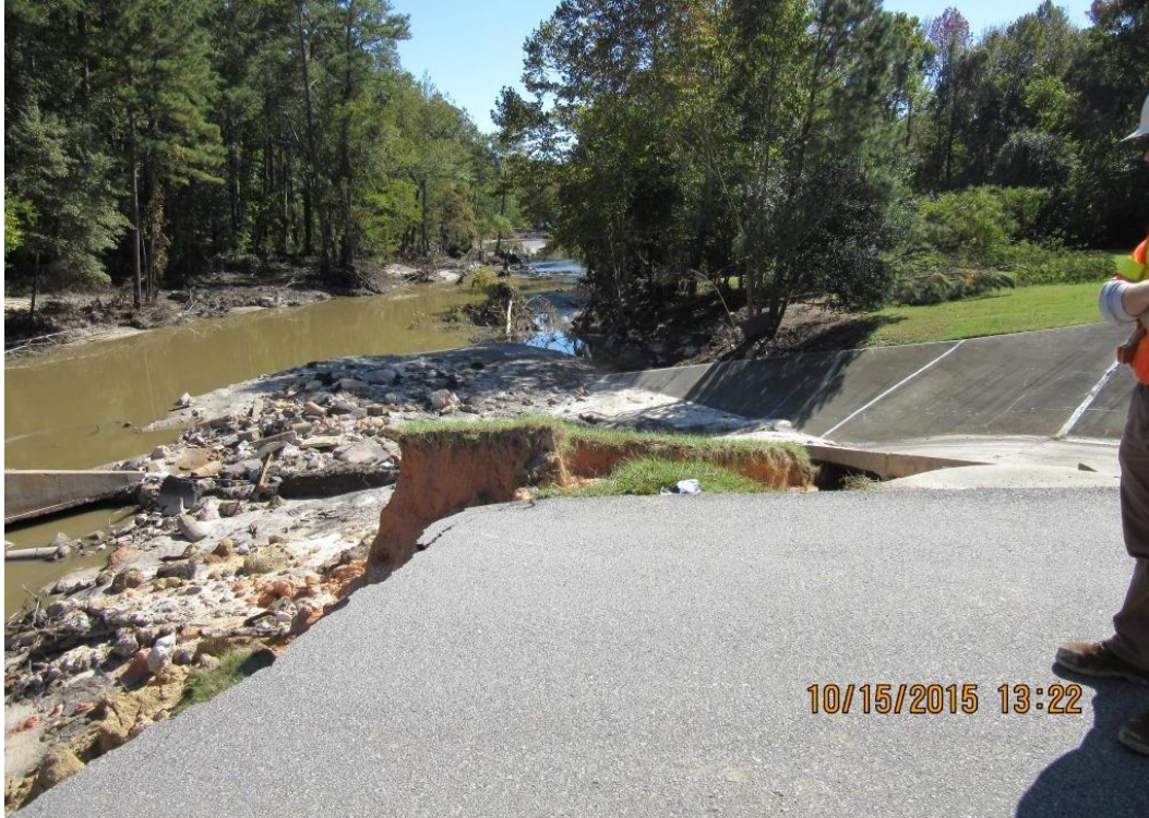
Photo 3: Downstream view of remnants of right concrete channel of the auxiliary spillway.
