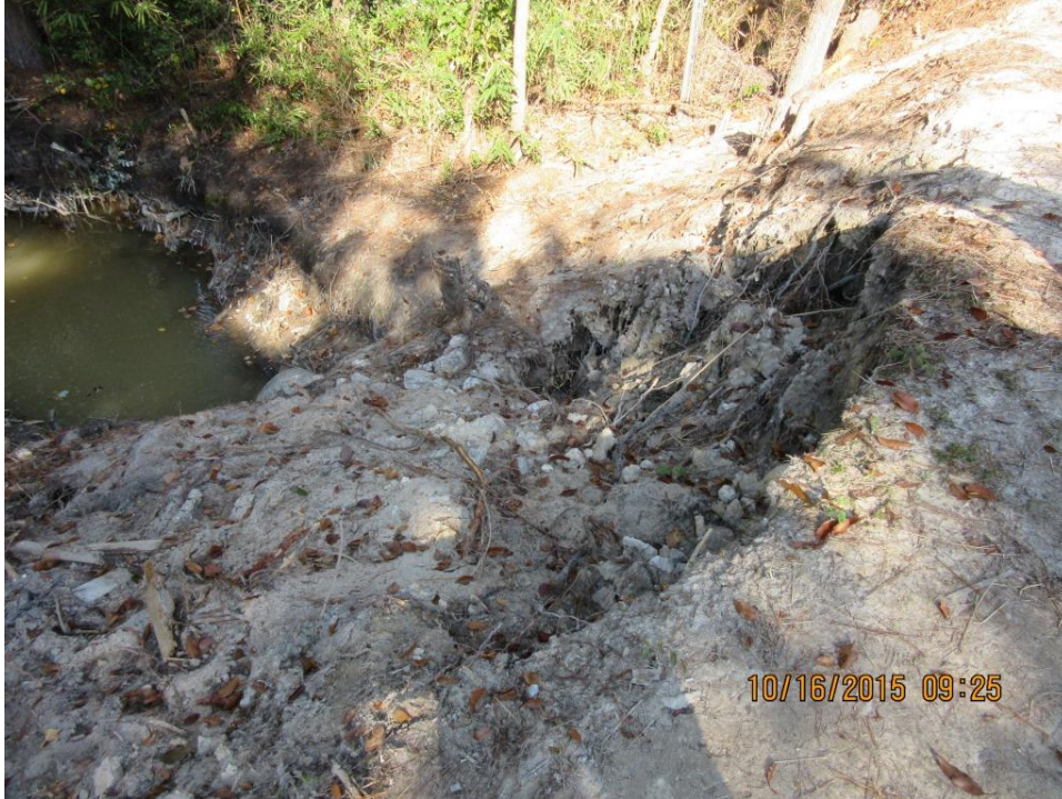
Photo 5: Slough of downstream slope viewed from embankment crest
