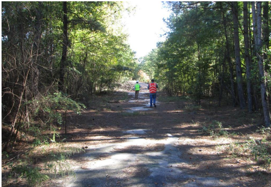
Photo 1: Crest of embankment dam looking toward the left abutment. Note mature trees and thick underbrush on embankment slopes.
