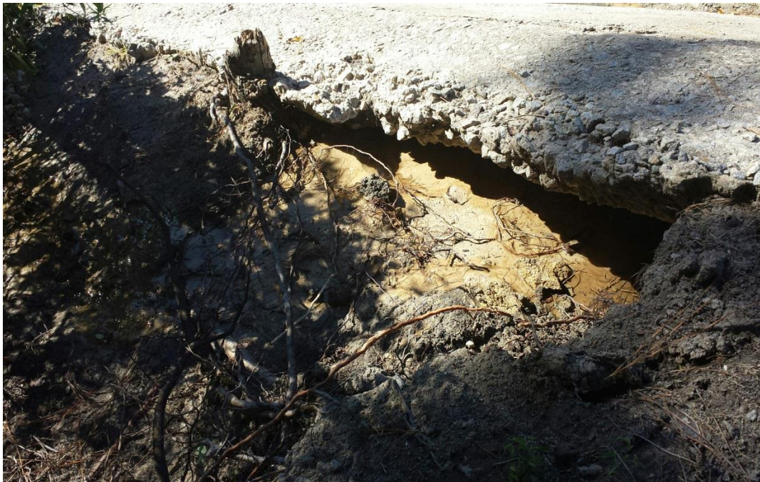
Photo 8: Undercutting and minor seepage along left side of auxiliary spillway concrete channel
