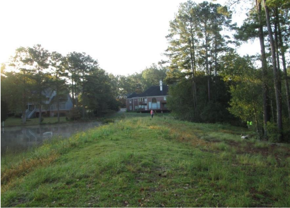
Photo 1: Embankment crest viewed from right abutment. Grass cover on upstream slope; trees and underbrush on downstream slope and toe.
