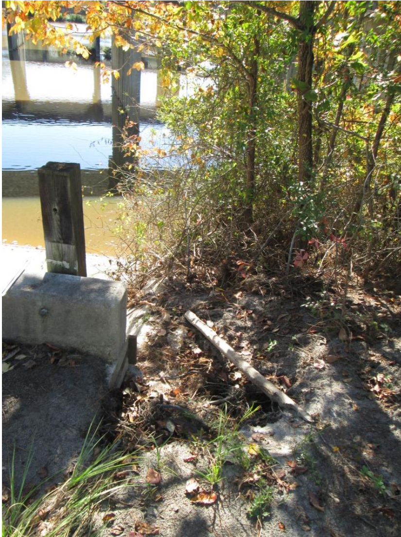
Photo 7: Erosion at auxiliary spillway/bridge right abutment
