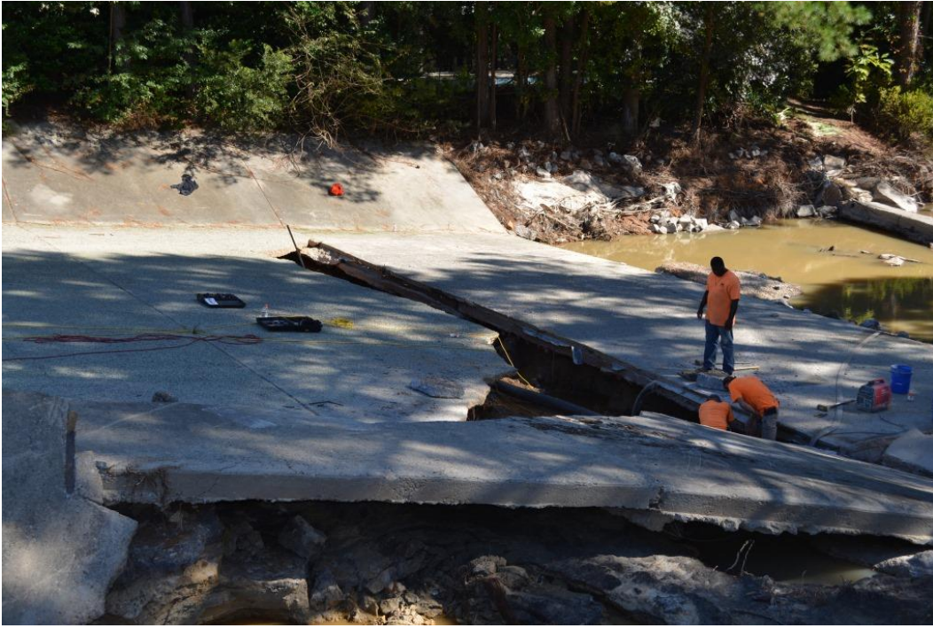
Photo 4: Auxiliary spillway damage
