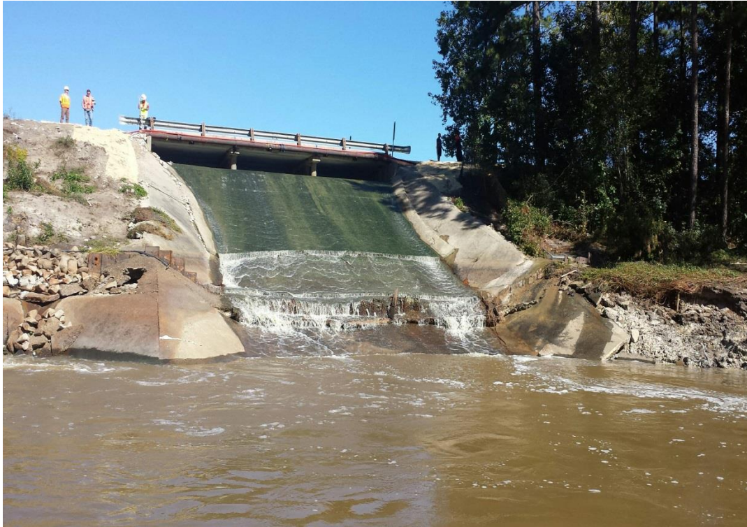
Photo 5: View of auxiliary spillway; note erosion at toe of left embankment
