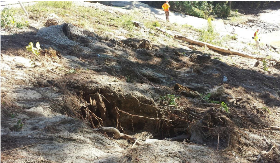
Photo 2: Erosion on downstream slope of the right embankment
