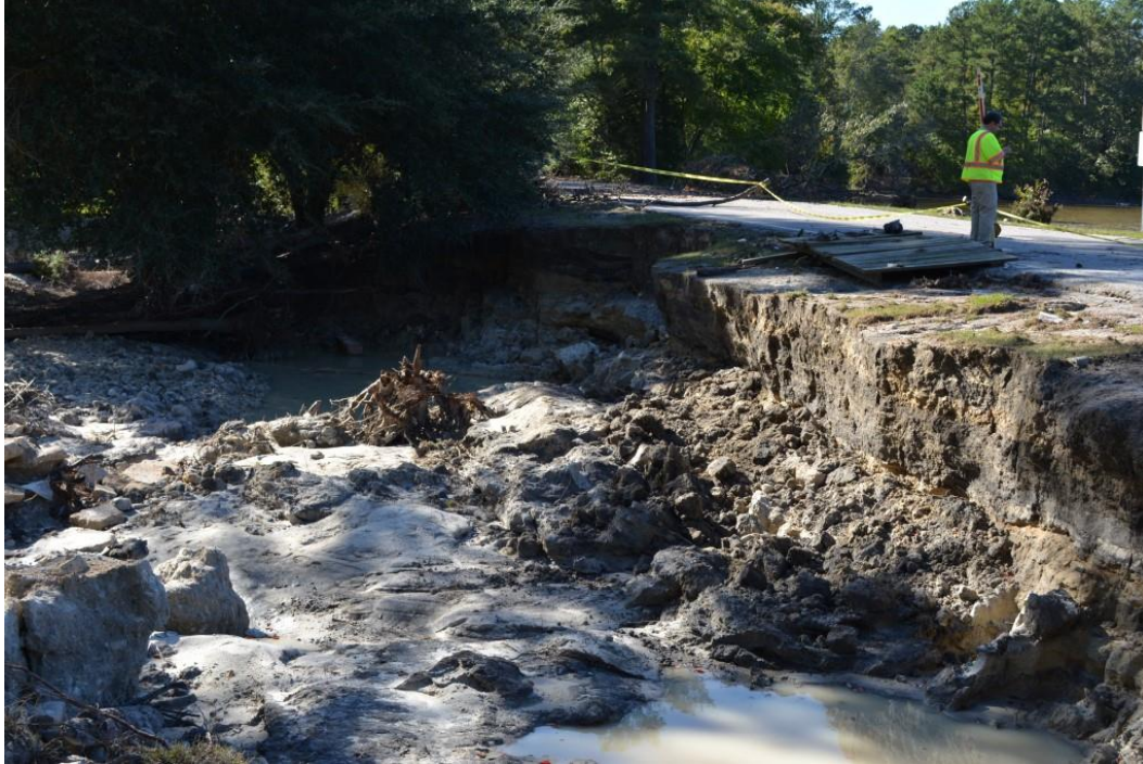
Photo 1: Erosion and headcutting of downstream slope of embankment dam
