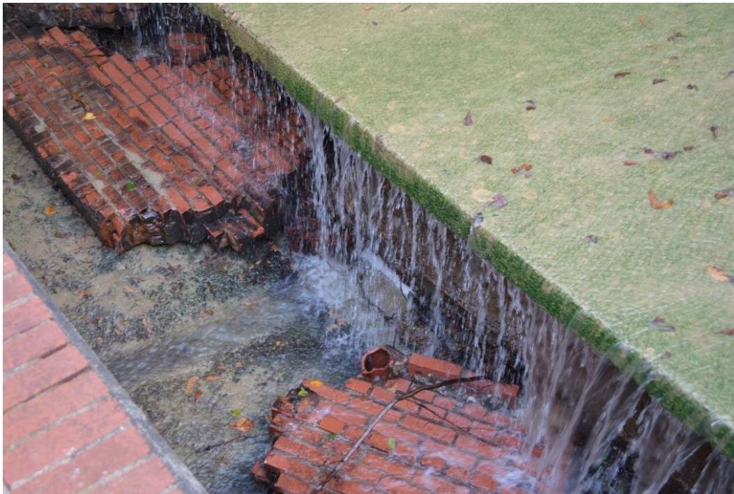
Photo 10: Damage at downstream end of auxiliary spillway
