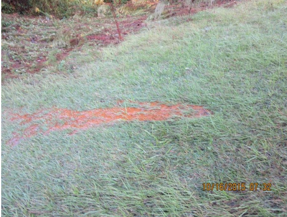
Photo 9: Seepage at downstream end of auxiliary spillway
