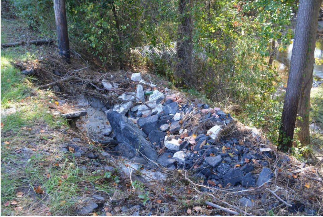
Photo 3: Downstream embankment slope erosion
