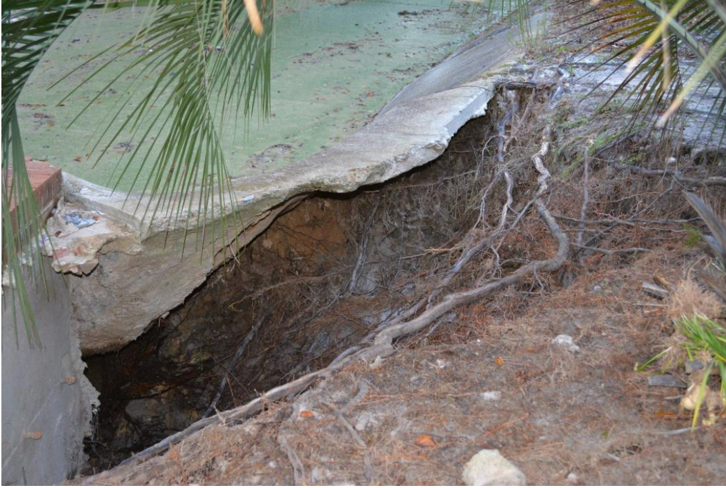
Photo 11: Erosion at end and left of auxiliary spillway
