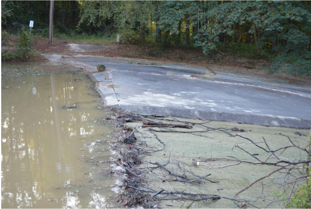
Photo 9: Auxiliary spillway with debris
