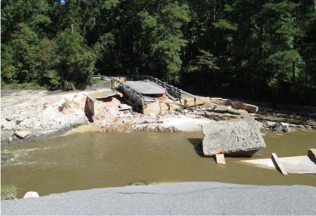
Photo 1: View of dam breach and left abutment from right abutment.
