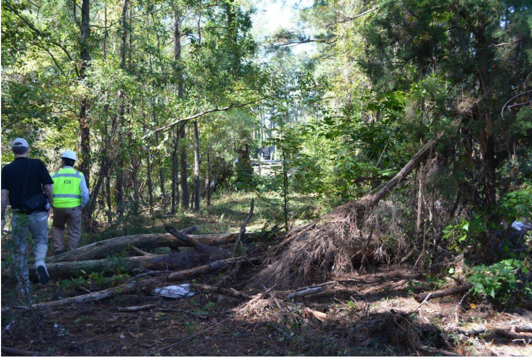
Photo 3: Right embankment crest looking toward right abutment showing tree growth on upstream and downstream slopes
