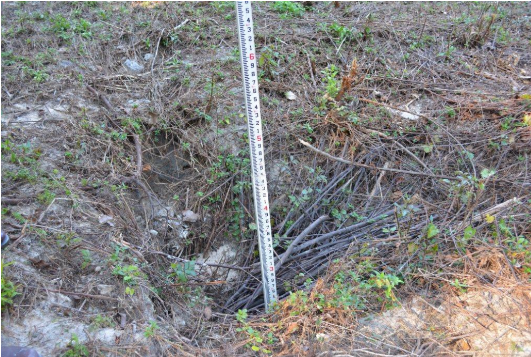
Photo 6: Depression at embankment toe along alignment of the service spillway outlet pipe
