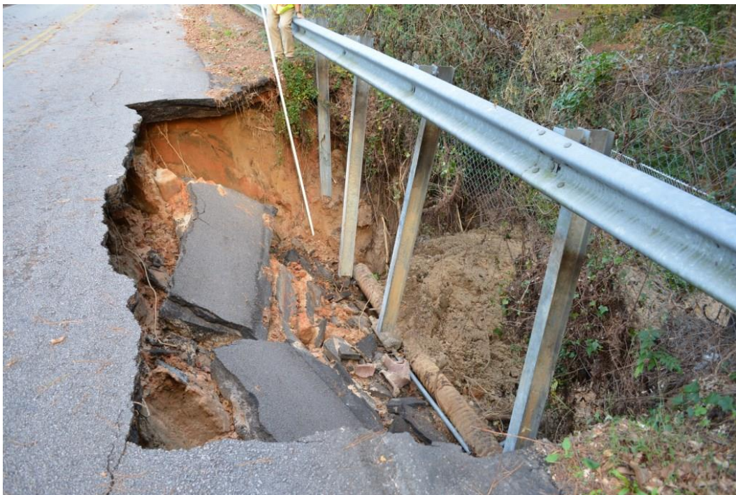
Photo 4: Slope failure on downstream slope of embankment
