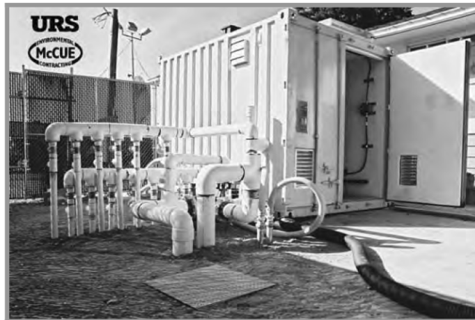
Photograph 2: Compound including equipment enclosure, SVE manifold, automated valve and piping, header connections and well roadbox.
