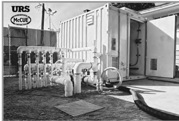
Photograph 2: Compound including equipment enclosure, SVE manifold, automated valve and piping, header connections and well roadbox.
