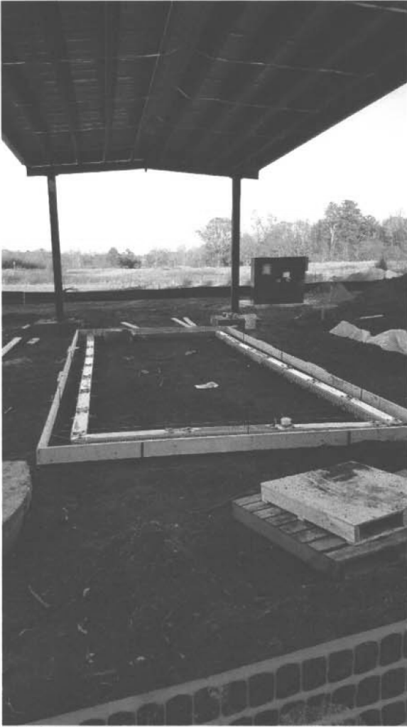
12/22/2016: Canopy frame is constructed and compressor pad is being framed for concrete pour.
