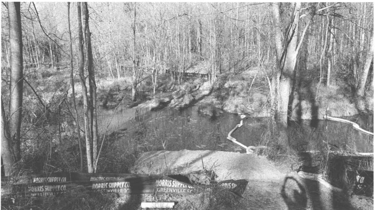
Reactive core mat and erosion control blanket installed at Seep 2 adjacent to Brown's Creek.
