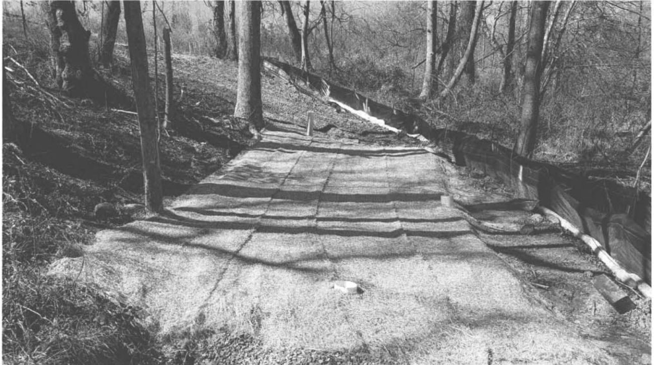
Reactive core mat and erosion control blanket installed at Seep 1 (Brown's Creek is just out of frame to the right of the photo).
