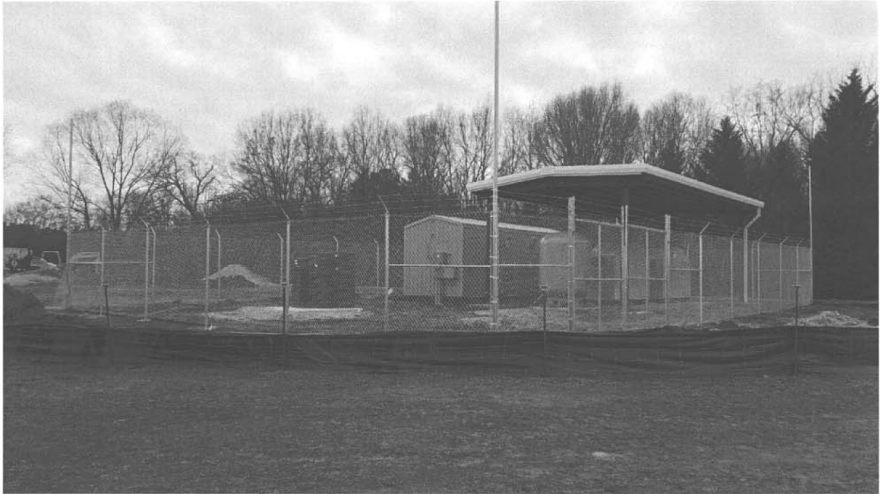
Equipment compound with fencing, lights, and gates
