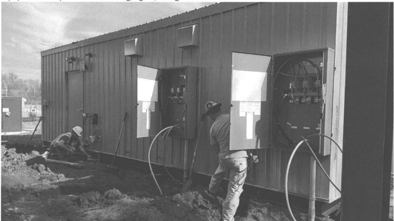
Electrical connection to compressor feeders
