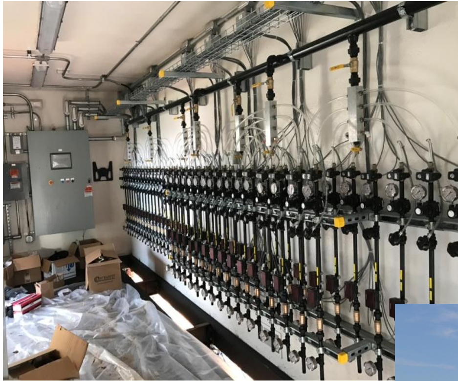
Biosparge Control Building- Interior
