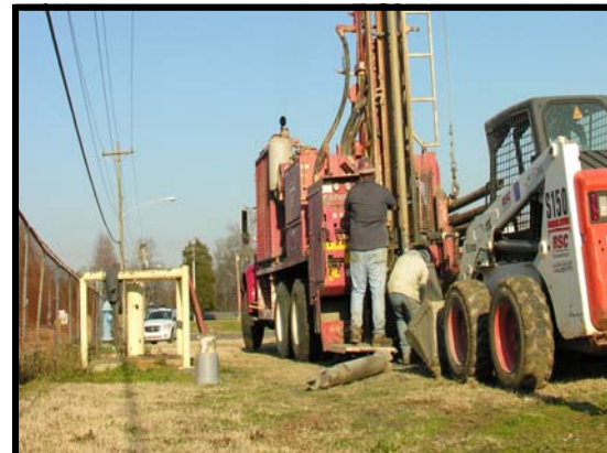
W1 (center yellow pipe left of rig)
