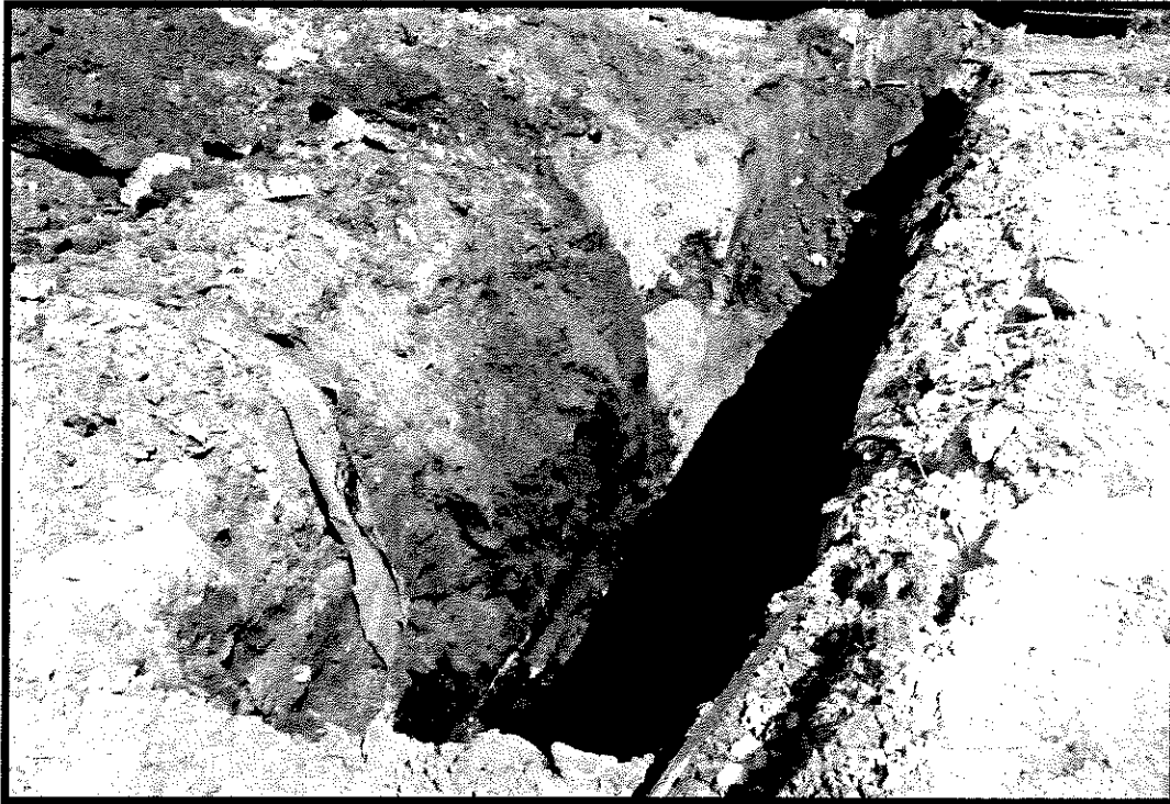
SDTP-8 with NAPL blebs on gravel above concrete "floor"
