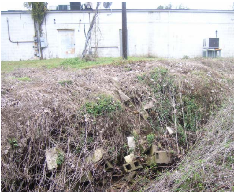
Figure G-6: Trash and debris in the stream and stream banks near station RS-01023
