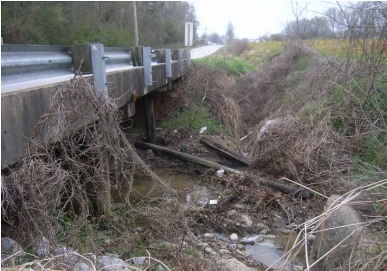
G-13: Railroad Avenue Bridge down stream of PD-258. Note the debris in the stream and stream banks.
