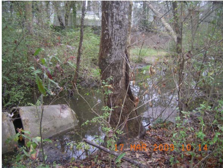
Figure G-5: Station RS-06027, on Ashby Branch. The picture below was taken while standing on the right bank of Ashby Branch depicts area downstream of Clark Street. Note the broken pipe.
