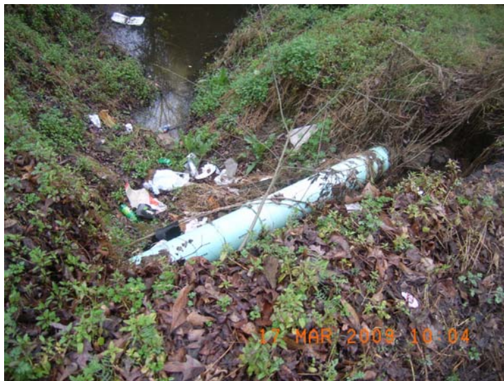
Figure G-1: Station RS-06027, on Ashby Branch. The picture below was taken while standing on Clark Street and depicts area upstream.
