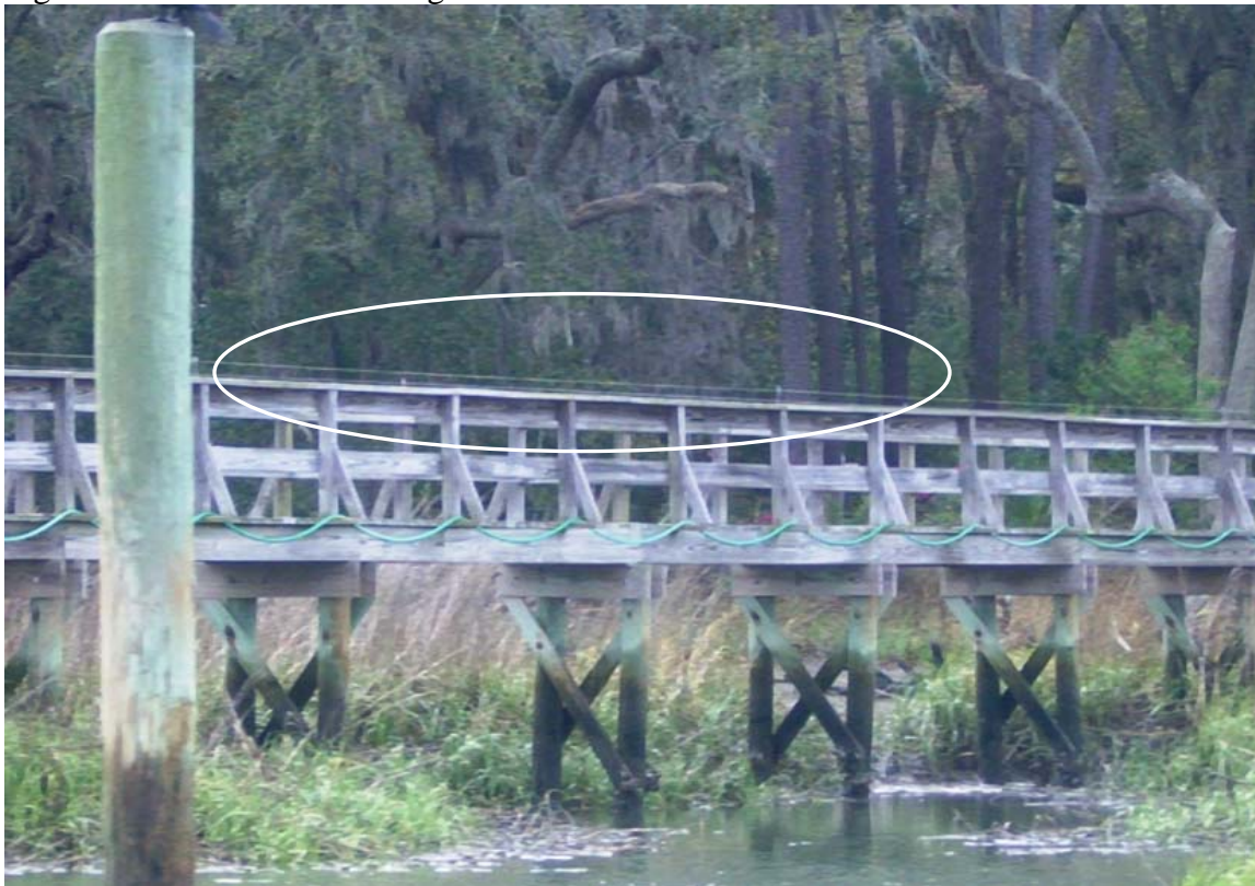
Figure 10. Bird deterring plastic coated wires on dock railings.
