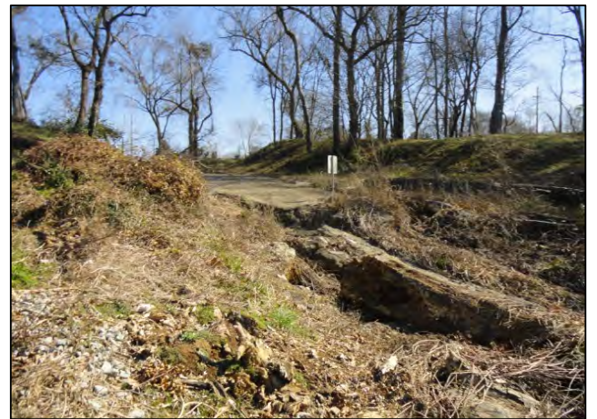
View of the end of Senate Street Extension from alluvial fan (Note eroded area that will require reconstruction)
