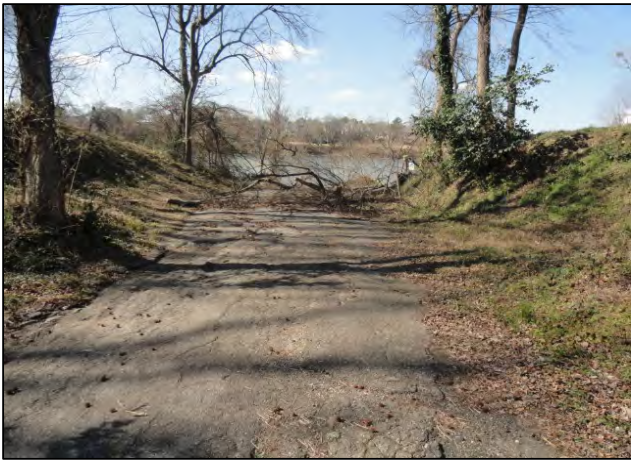
Senate Street Extension looking towards alluvial fan (Note tree limbs requiring removal)
