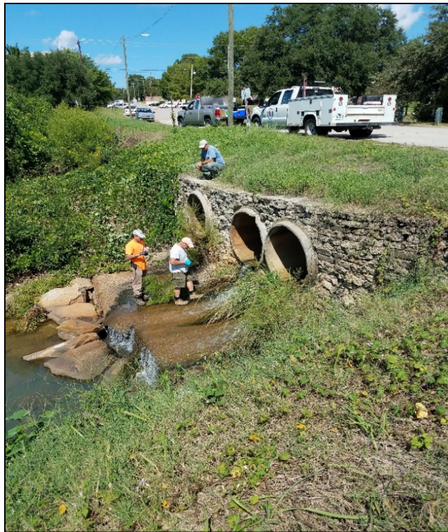
Memorial Park Outfall - SW-01 (Typical)
