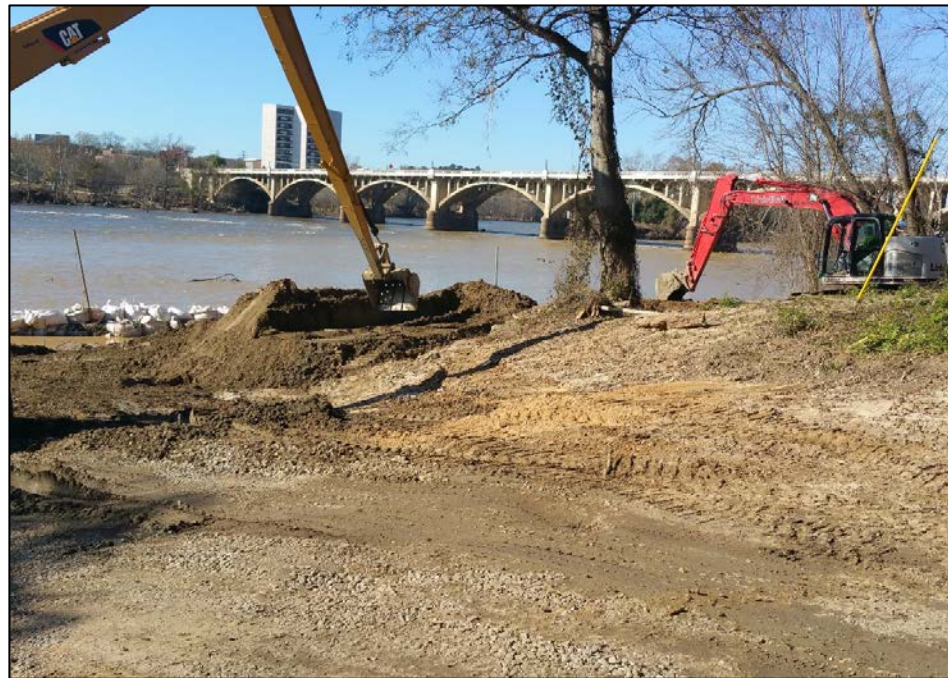
12/07/2015 - Placing removed sediment back on alluvial fan surface and restoring to post-flood elevations
