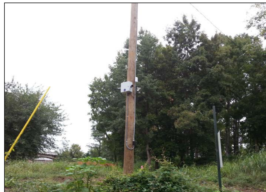
9/28/2015 - Security cameras overlooking the FDP area
