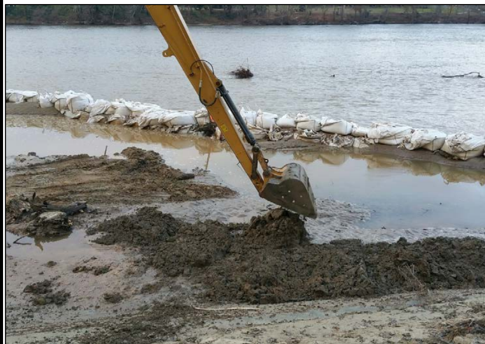
12/07/2015 - Placing removed sediment back on alluvial fan surface and restoring to post-flood elevations
