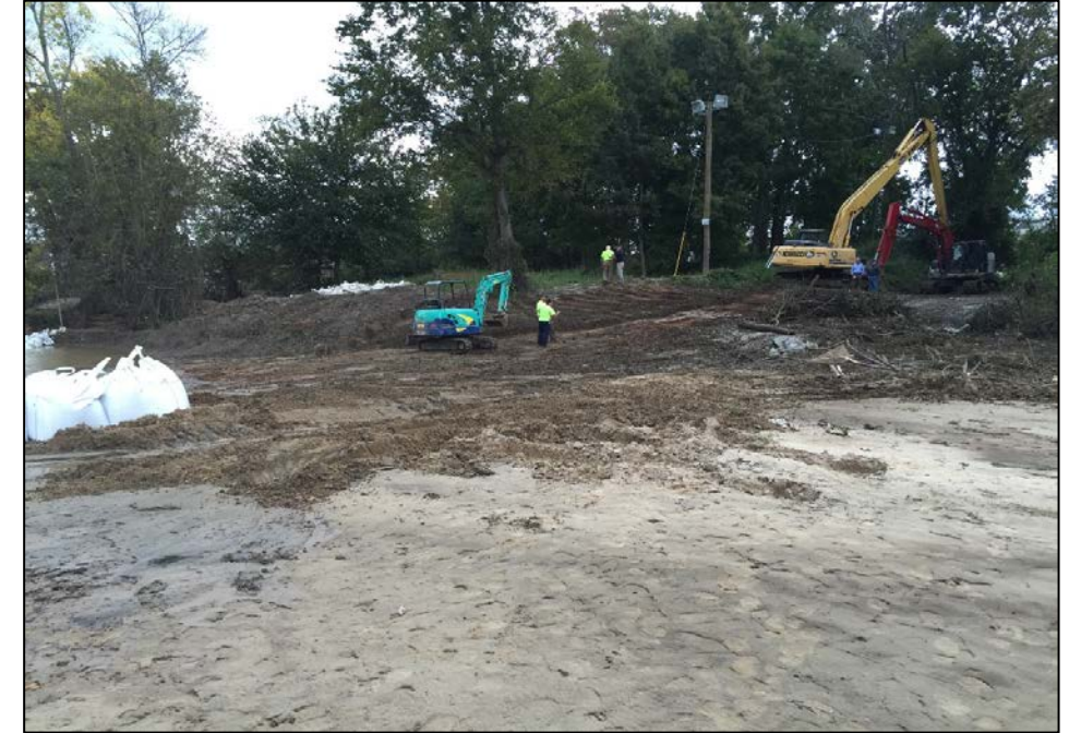
10/28/2015 - Sediment deposited by flood event removed and alluvial fan restored to pre-flood elevations
