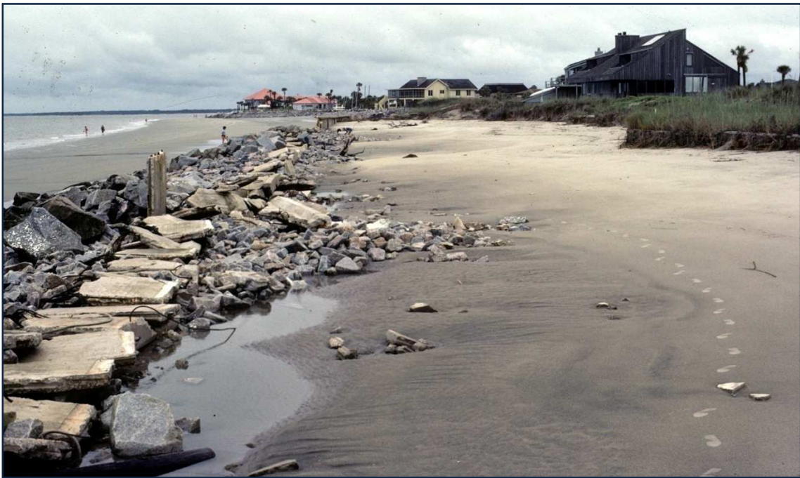
FIGURE T-8. [UPPER] Encroachment of the northern channel (deep blue area) of North Edisto Inlet and lack of maintenance leads to [LOWER] collapse of a section of seawall near Beach Court in 1983.
