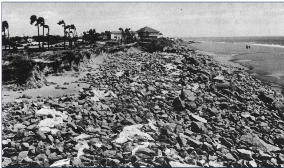
FIGURE 5.2.3a. Damages along Seabrook Island due to Hurricane David (5 September 1979). [UPPER] The concrete seawall and armor-stone “wingwall” at Renken Point on 7 September 1979. [LOWER] Collapsed riprap revetment south of the Beach Club on 5 September 1979. [Photos by WJ Sexton]
